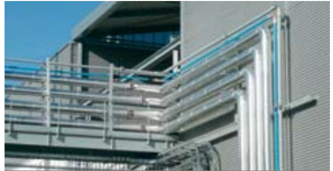
Outdoor installation Transair Ø 168
